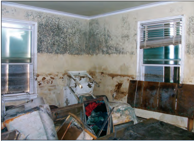
Figure 6. Mold and biological/chemical contamination are also concerns when flood levels rise above the lowest floor. Contamination may result in the building being irreparable or, at least, make the cleanup, restoration, and repairs more expensive and time-consuming.
