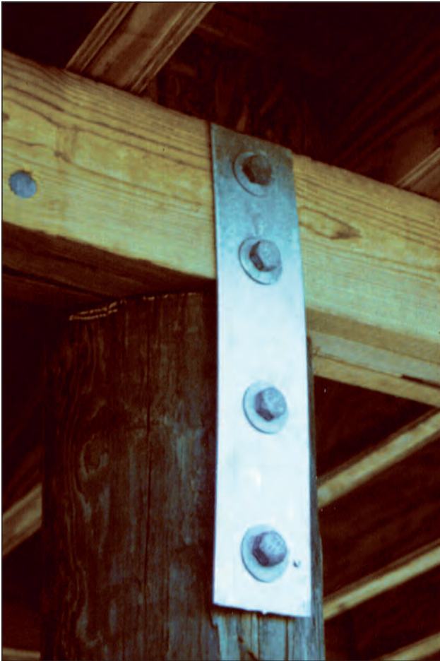
Metals corrode at a much faster rate near the ocean. Always use well-protected hardware, such as this connector with thick galvanizing. (For information about pile-to-beam connections, see Fact Sheet No. 3.3, Wood Pile-to-Beam Connections.)
