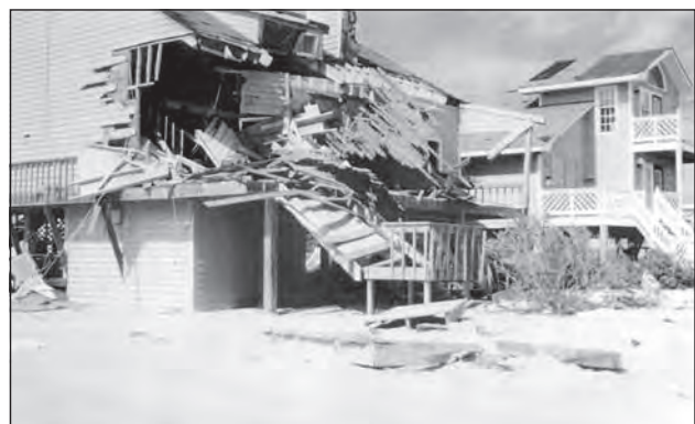
Figure 2. Well-sited building that still sustained damage.
