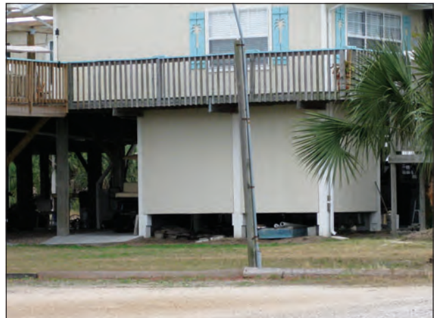
Figure 6. Example of an enclosure that does not extend to grade. This type of enclosure presents special construction and flood insurance issues. Contractors should proceed with caution when an owner requests such an enclosure.
