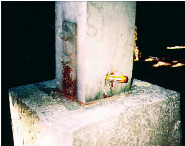
Wood decay at the base of a wood post supported by concrete.
