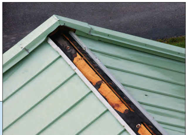
Figure 9. The ridge flashing fasteners were placed too far apart. A significant amount of water leakage can occur when ridge flashings are blown away.
