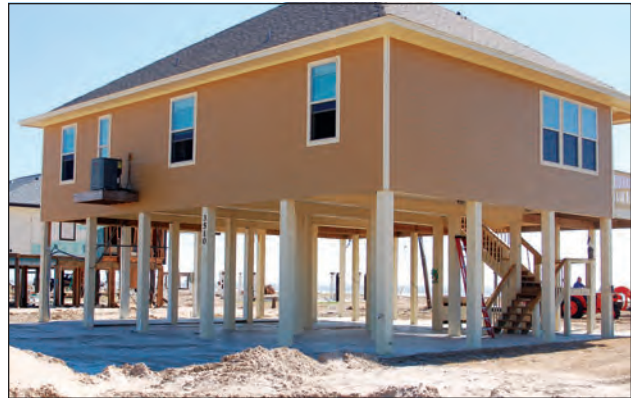
Figure 2. Breakaway walls beneath this building failed as intended under the flood forces of Hurricane Ike.
