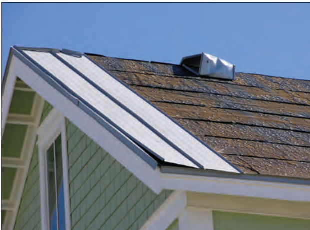
Figure 3. These architectural panel system have snap-lock seams. One side of the seam is attached with a concealed fastener. Although a large number of panels blew away, the underlayment did not.
