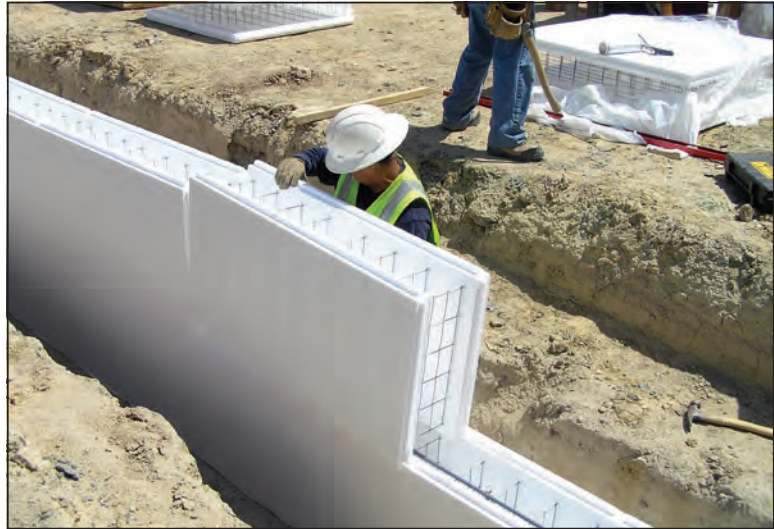
Figure 3. An example of ICF walls and reinforcing steel prior to placement of the concrete. The forms are left in place following placement of the concrete.
