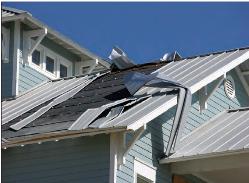
Figure 2. This architectural panel system has concealed clips. The panels unlatched from the clips. The first row of clips (just above the red line) was several inches from the end of the panels. The first row of clips should have been closer to the eave.
