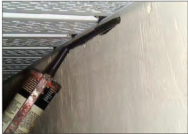
Figure 3. Applying a bead of sealant. (Note: Black sealant was used so that it would be visible in the photograph. Normally a matching sealant color would be used.)
