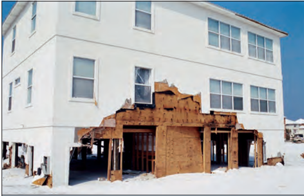
Figure 4. Building siding extended down and over the breakaway wall. Lack of a clean separation allowed damage to spread upward as the breakaway wall failed.
