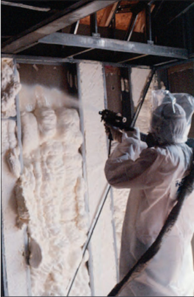
Figure 5. An example of a wall cavity filled with sprayed closed-cell foam insulation.
