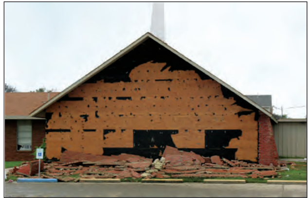
Figure 1. Failed brick veneer over plywood. Many of the ties are still attached to the substrate, but several of the tie fasteners pulled out of the substrate and the ties are embedded in the collapsed veneer. Estimated wind speed: 107 miles per hour (peak gust, Exposure C, at 33 feet).
