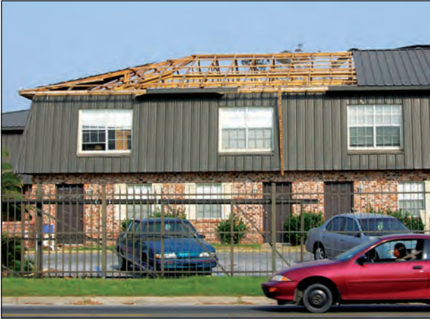
Figure 6. Blow-off of nailers caused these panels to progressively fail. The nailers were installed directly over the trusses. In an assembly such as this where there is no decking, there is no opportunity to incorporate an underlayment. With loss of the panels, rainwater was free to enter the building.
