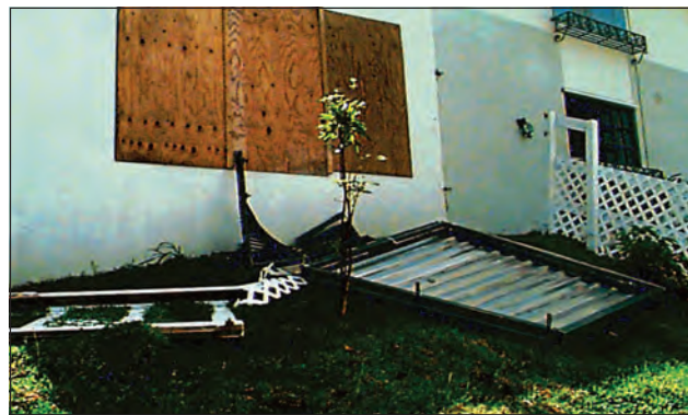
Figure 3. Hurricane Georges in Puerto Rico. The window lying on the ground was protected by a shutter. However, the shutter was attached to the window frame. The window frame fasteners were over-stressed and the entire assembly failed. Attachment of the shutter directly to the wall framing is a more reliable method of attachment.
