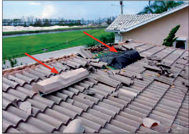
Figure 11. Two off-ridge vents are shown in this photograph. The vent that is covered with roofing felt flipped up and allowed a substantial amount of water to enter the residence. Carpeting, kitchen cabinets, and a large amount of gypsum board had to be replaced because of the water intrusion.
