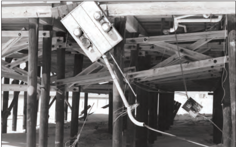
Electrical lines and box dislocated by hurricane forces.
