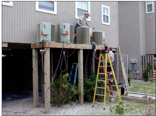
Elevated air conditioning compressors.
