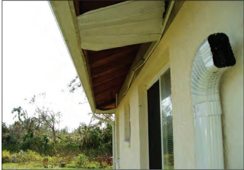
Figure 1. Missing soffit material.
