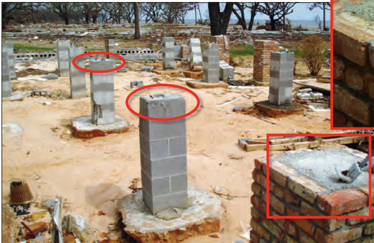
Figure 3. Failure of pier-to-beam connections due to wave and flood forces acting on the elevated building (Long Beach, Mississippi)
