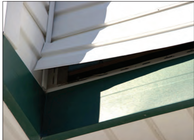
Figure 4. Utility trim was substituted for the starter strip and the bottom lock was cut off the siding. Siding was able to pull loose under wind pressure.
