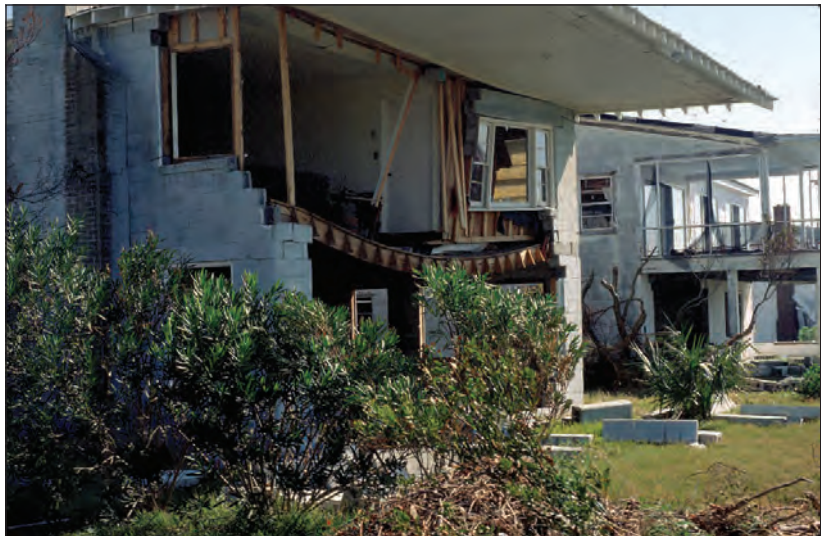
Figure 1. Storm-damaged homes need repairs, but also provide opportunities for renovation, additions, and retrofitting. Review substantial damage and substantial improvement regulations before undertaking any work.
