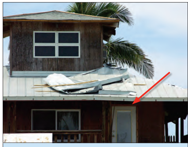
Figure 5. The panels blew off the upper roof and landed on the lower roof of this house. The upper asphalt shingle roof shown had been re-covered with 5V-Crimp panels that were screwed to nailers. The failure was caused by inadequate attachment of the nailers (which had widely-spaced nails) to the sheathing. Note that the hip flashing on the lower roof blew off.
