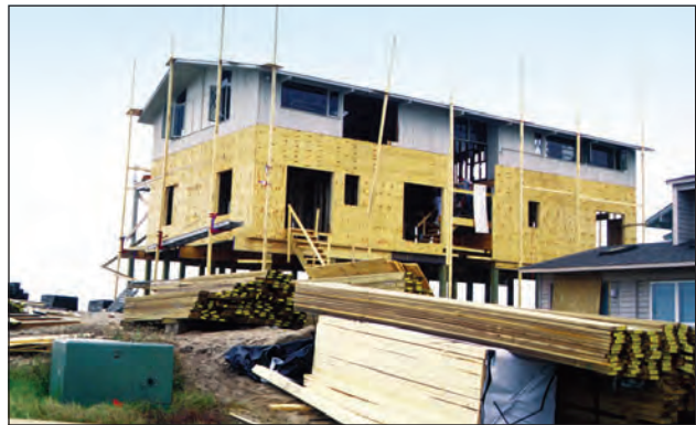
Figure 2. Vertical addition to a home damaged by Hurricane Fran. Preexisting 1-story home became the second story of a home elevated to meet new foundation and floor elevation requirements.
