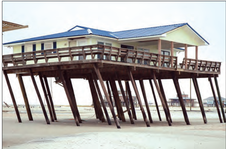
Figure 1. Near collapse due to insufficient pile embedment in Dauphin Island, Alabama.
