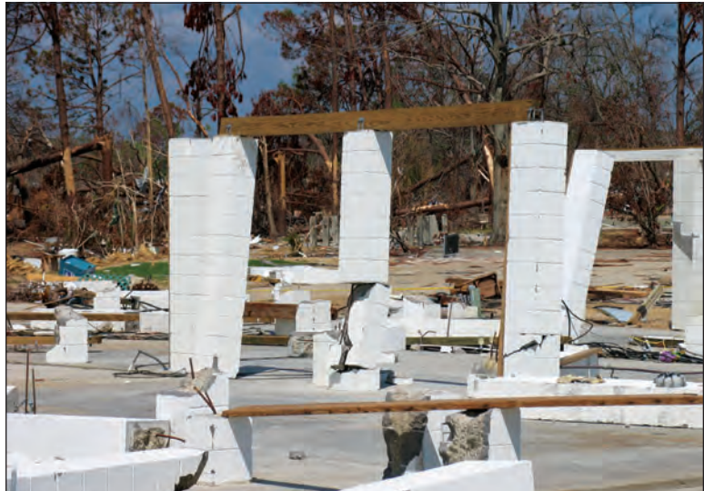
Figure 2. Pier breakage (Long Beach, Mississippi)
