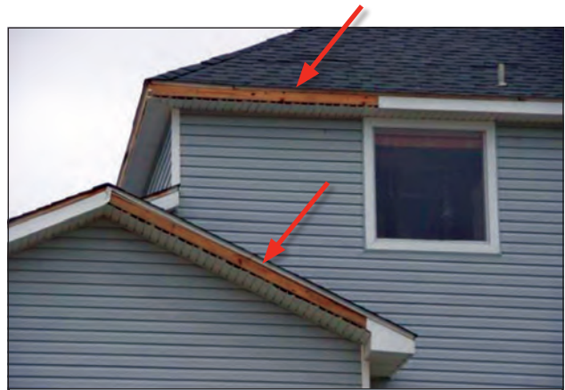
Figure 7. Loss of fascia cover exposes ends of vinyl soffit to direct entry of wind-driven rain.
