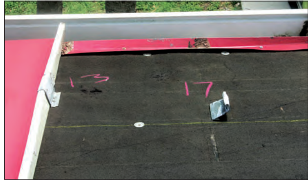
Figure 4. These eave clips were too far from the panel ends. The clip at the left was 13" from the edge of the deck. The other clip was 17" from the edge. It would have been prudent to install double clips along the eave.
